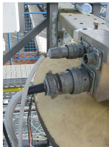
(b) Cable deterioration
